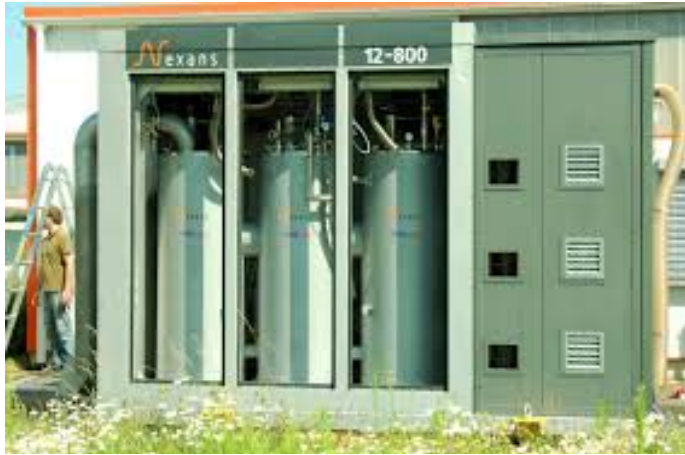
Fig 6.1 SFCLs installed for distribution level
