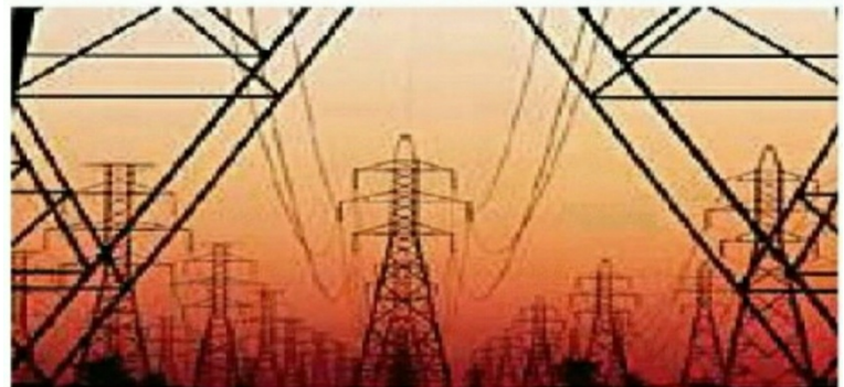
Fig 3.1 Compact Arrangement Of Transmission Lines
